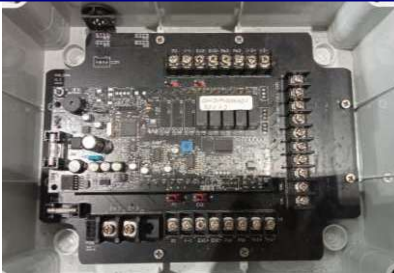
COMPUTER BOX WITH SWITCHES FIG. 3-9
